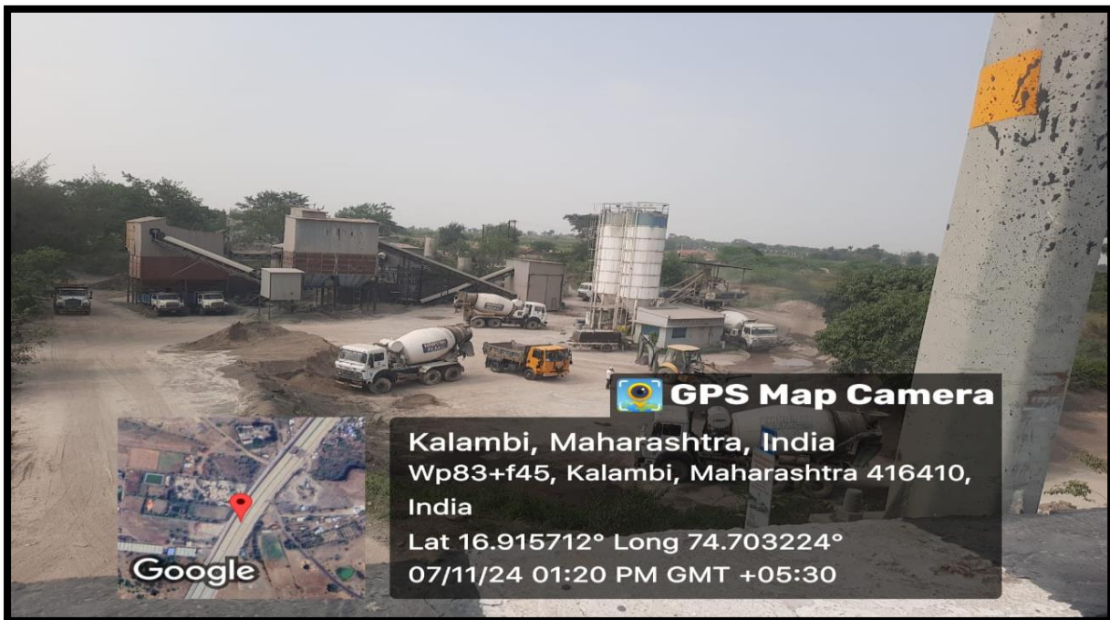
Pictures dated 07.11.2024 showing that RMC unit of Respondent No. 2 is operating illegally.
